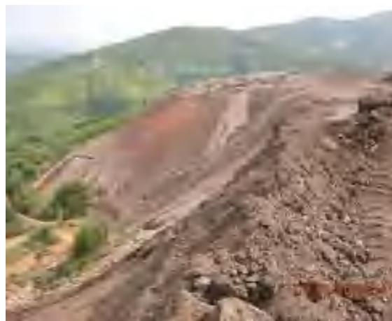
治理前矿渣堆边坡
